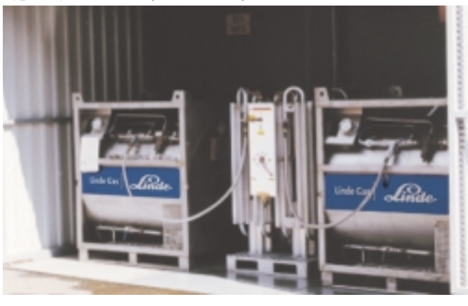
Figure 15: Liquid Nitrogen Stored in a Pallet Tank Holds Typically 600 Liters (300 Gallons) of LIN
